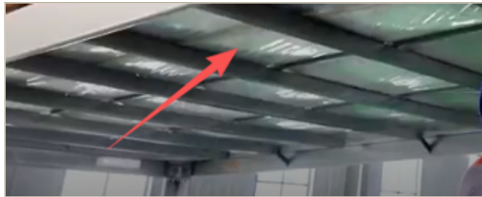
FIG. 5.1 Plastic sheet (CH-FAS-019015) laid over the secondary beams and held down with double-sided tape — view from below.
